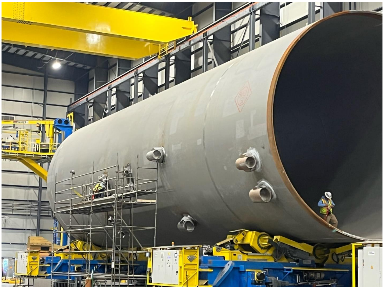
A welder on steel scaffolding and a second worker inside the mouth of a monopile section in the Circ Weld Building are dwarfed by the massive monopile section.
